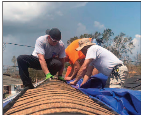
Hurricane Ida Response Louisiana
