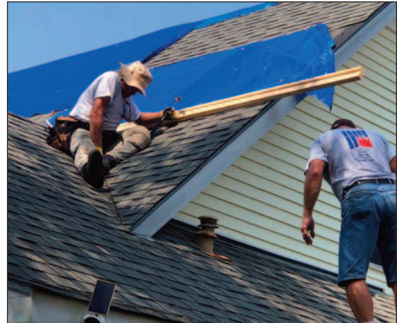
Hurricane Ida Response Louisiana
